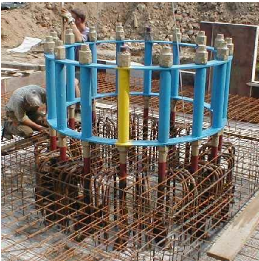
Figure 2 Anchor cage built in on construction joint, yellow marking on axis of exhaust gas inlet. The cap bracket and the lightning protection grounding have been arranged on the lower armouring unit which cannot be seen in the figure. The upper armouring will still have to be completed.
