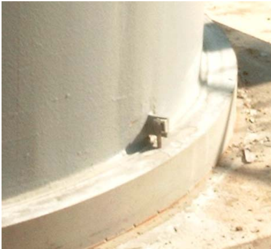
Figure 4 Readily grouted chimney base with ground connection.
